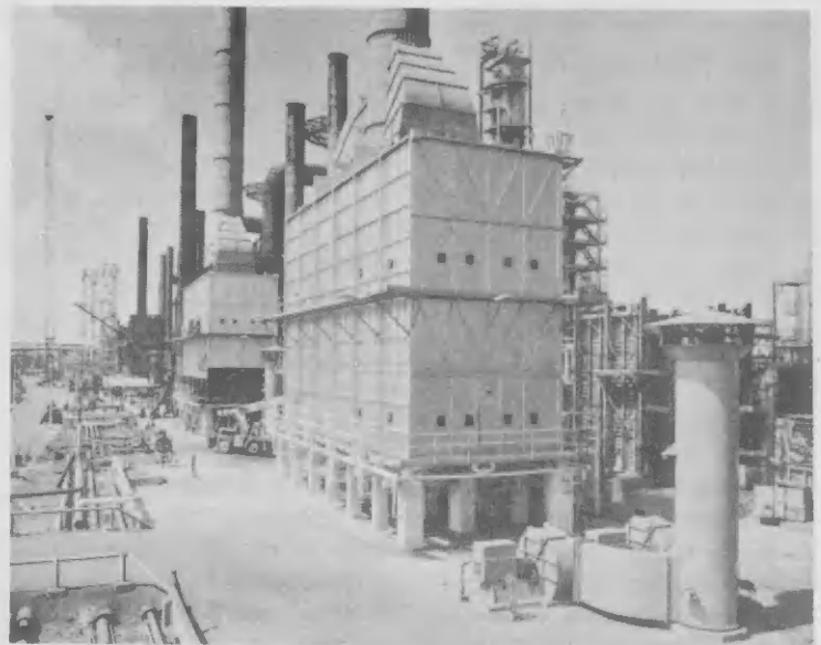
This new furnace for No. 8 Pipestill (in foreground) was placed in service Jan. 24. In background is the furnace of Pipestill No. 7, while the new furnaces for Pipestill Nos. 6 and 5 are scheduled for completion in April.
